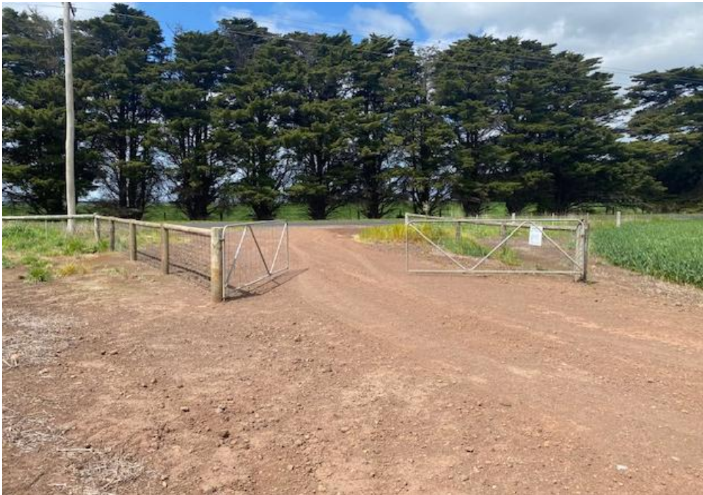
Indented gateway to be increased in depth to 20m. to allow off road truck parking.
