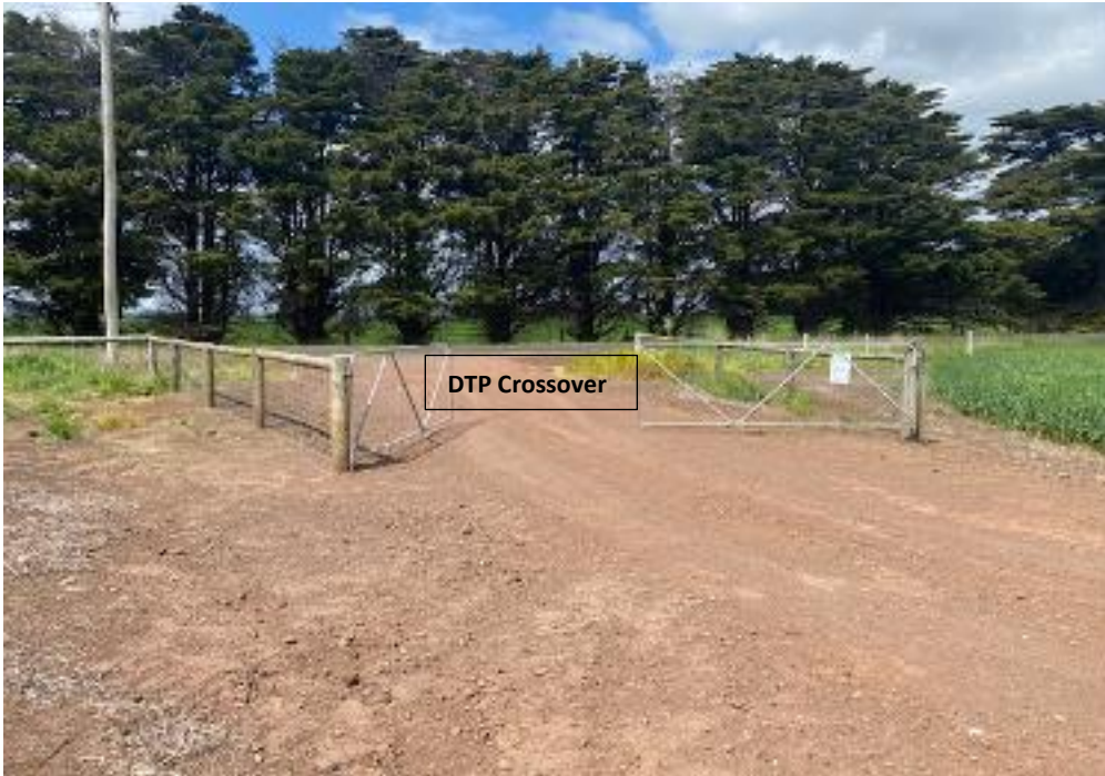
Existing Haul road entry gates. The haul road will be widened to 10m at the entry for a length of 40m and the gates moved 20m further into the haul road, this 20m section from the crossover to the gates will be sealed.
