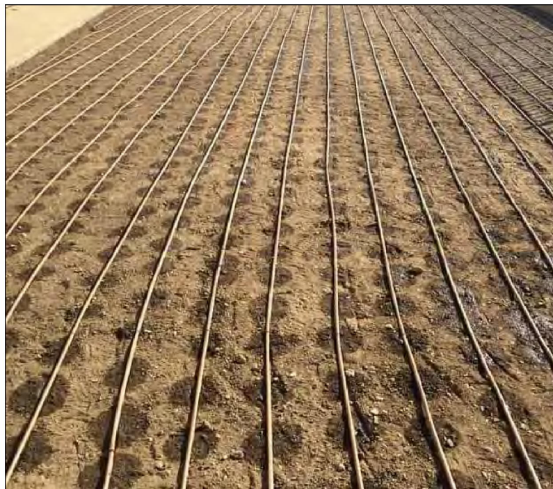
Figures 35-37 – Subsurface irrigation site preparation and piping network; flush valve (Source: Aquascope 2024).
