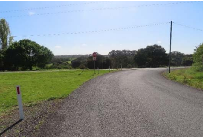
MORTLAKE-ARARAT ROAD & HEXHAM-WOORNDOO ROAD INTERSECTION FOR EAST BOUND TRAFFIC FACING STOP SIGN.
