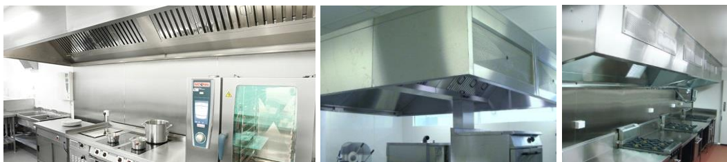
Figures 29-31 – Exhaust hoods shall be provided with approved metal washable dry type grease filters.
